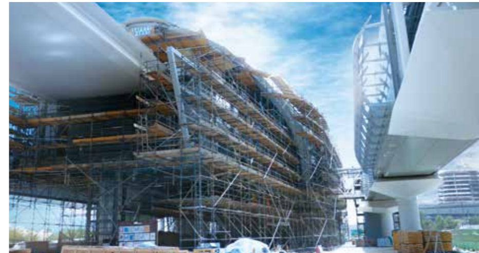
Project : Dubai Metro Client : Japan Turkey Metro Joint Venture Location : Al Jafiliya typical to all 15 stations Scope : Internal and External Access Scaffold for all the Stations and Depot
