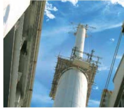
Project : DMCC Al Mas Tower Client : Jaggard Middle East Location : Dubai Scope : Cradle Rigging and Access for Antenna Installation
