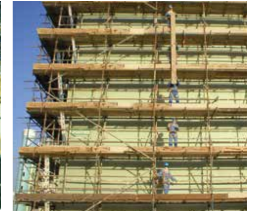
Project : Discovery Gardens Client : Larsen & Toubro Location : Dubai Scope : External Access Scaffold Painting Works
