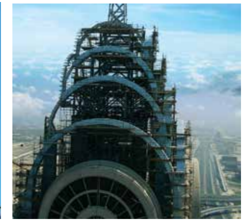
Project : Churchill Tower Client : Arabian Aluminum Location : Dubai Scope : Access Scaffold for Roof Feature
