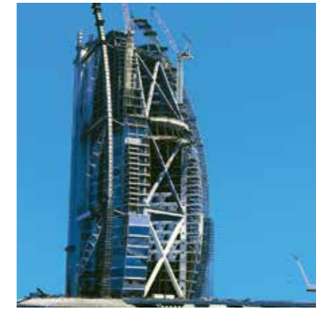
Project : Burj Al Arab Client : Arabian Aluminum Location : Dubai Scope : Temporary Suspended Access Platform on a Climbing Scaffold Rigging
