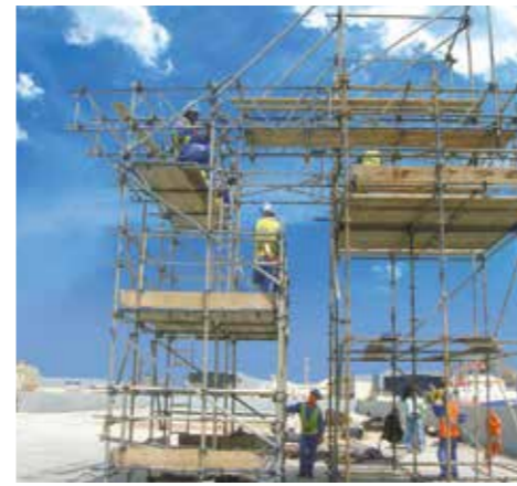
Project : Dredging & Land Reclamation Upper Zakum Artificial Islands Client : National Marine Dredging Co Location : Abu Dhabi Scope : Suspended Cantilever Access Scaffold for Quay Wall Furniture Installation
