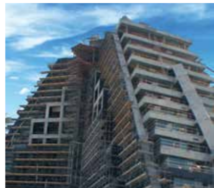
Project : Raffles Hotel - Dubai Client : Khansaheb Civil Engineering Location : Dubai Scope : External Access Scaffold for Cladding Works
